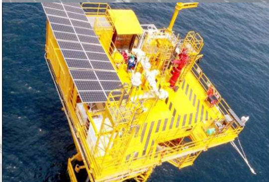
PLTS Off Shore 5 KWp
